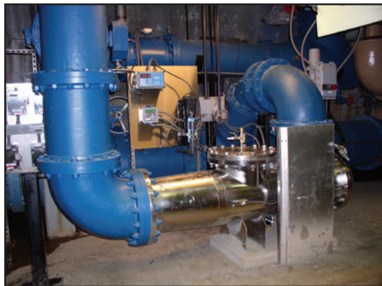
Figure 1. Poughkeepsie UV Disinfection System
