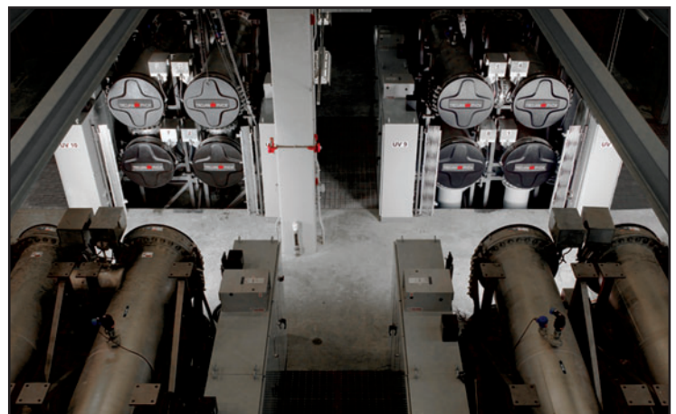
Figure 4. UV advanced oxidation at the Peter Binney Water Purification Facility
