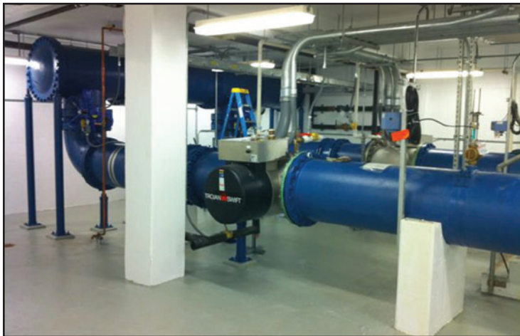
Figure 2. KPU's UV Disinfection System
